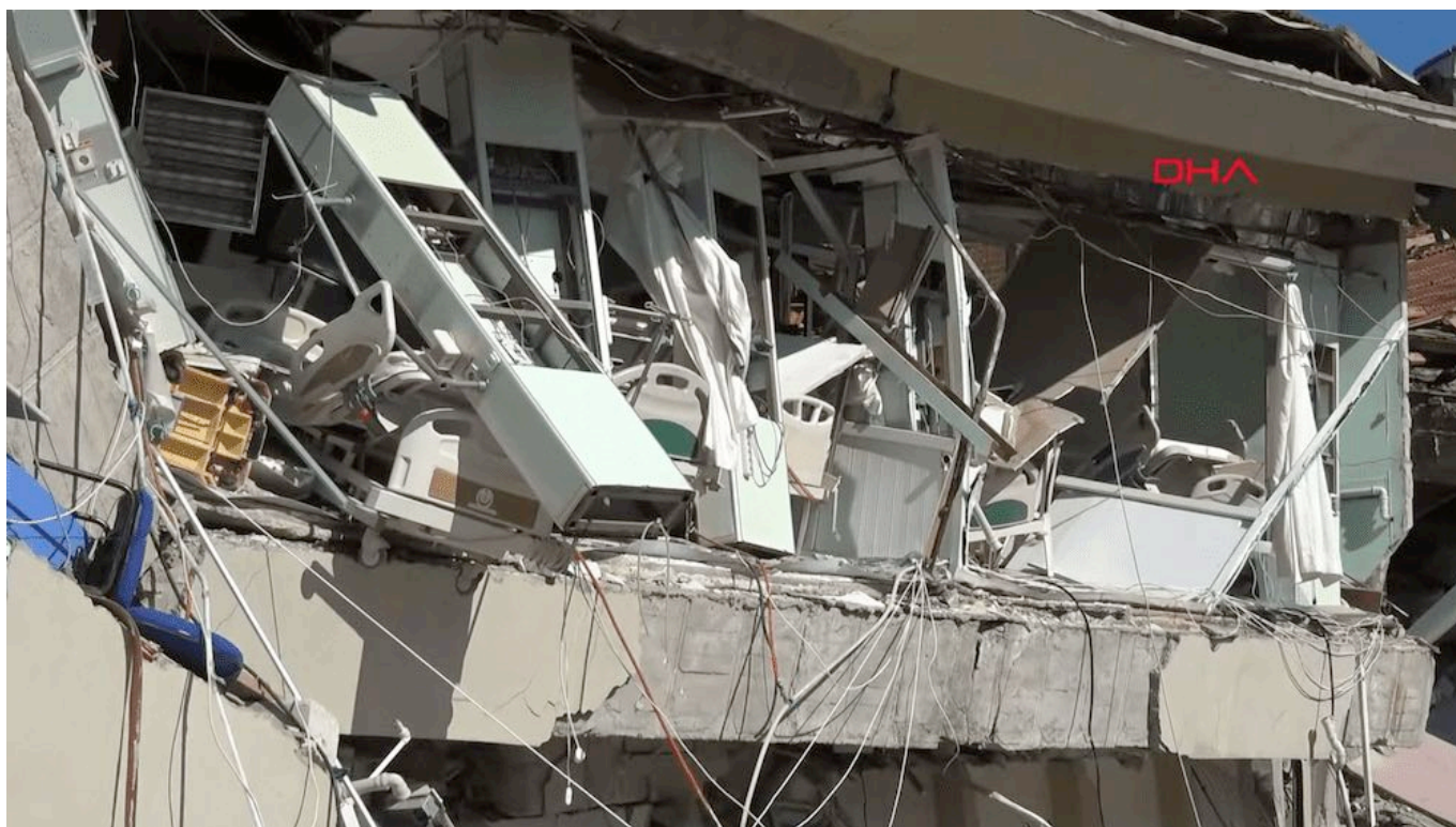
Hospital beds tip over the edge in part of the Hatay Education and Research Hospital in Antakya, which collapsed in the earthquake.
